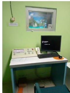
Figure 2 Computer Console Monitor (Radiology Installation of Sleman Hospital)
