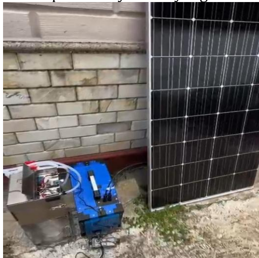
Gambar 3. Solar PV Charger Station System
